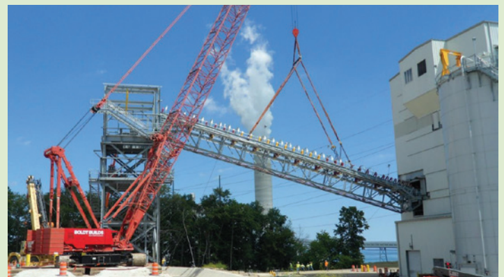
A crane lifts a conveyor truss from a transfer tower to a drive tower at Elm Road Generating Station.
